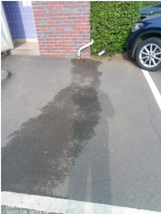
Drains blocked by the male toilets
