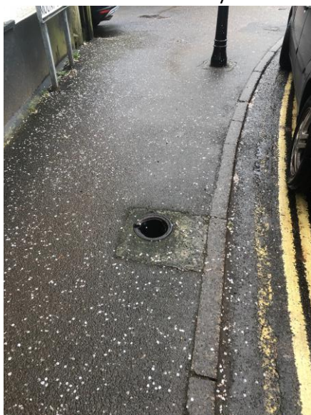
Bollard broke off by the Co op
